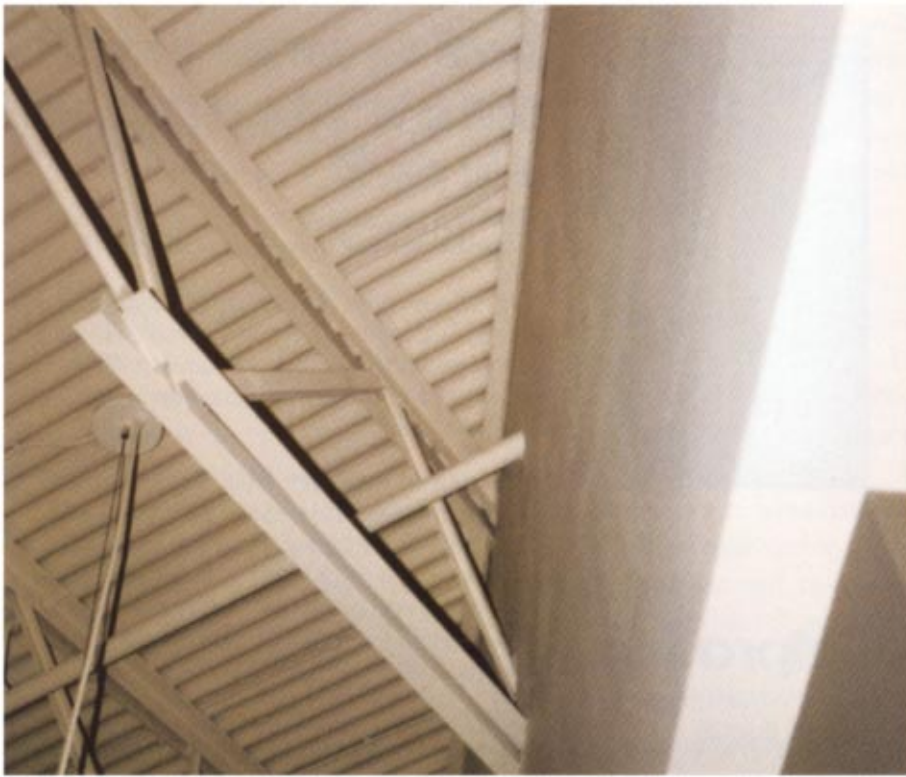
Finish around the joists of the Sav-A-Lot structure
