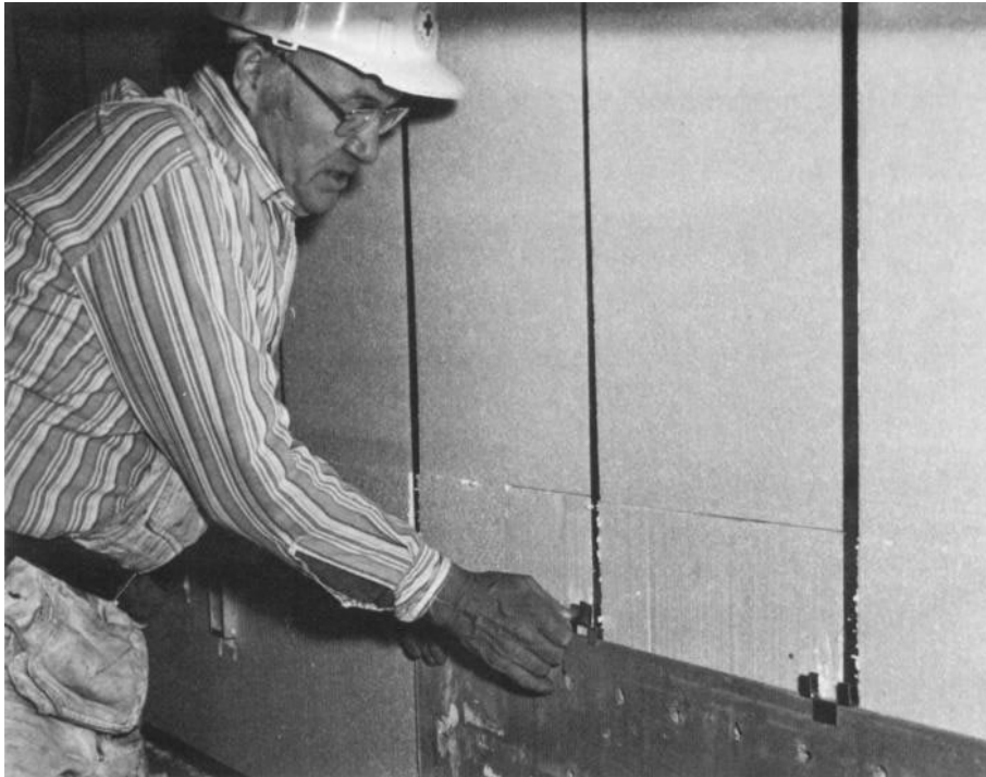
With all insulation in place, lath board or drywall panels are secured to expose Z-furring flanges. Screws or standard clipping hardware work equally well.
