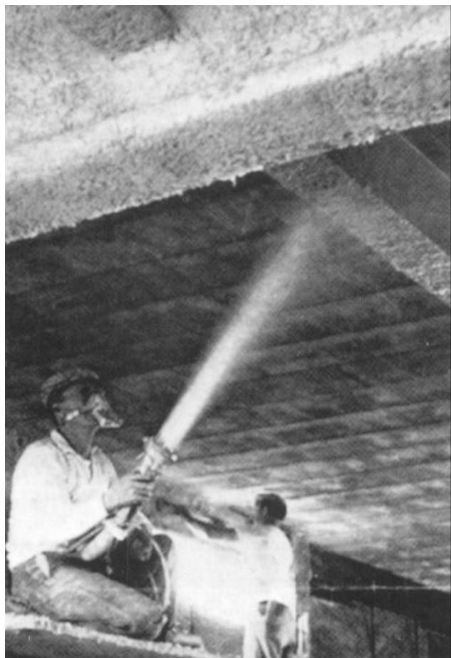
Mineral fiber fireproofing material is spray applied to steel decks, columns and girders.
