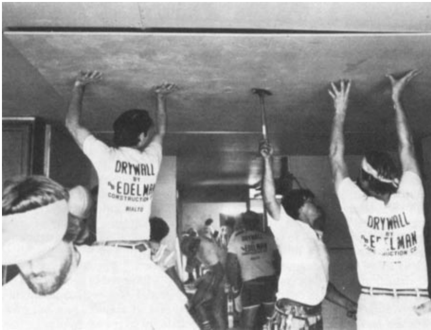
Dozens of workers on the "Drywall" team quickly yet carefully fit ceilings and walls into place during the recent "Woodhaven Challenge" initiated by Woodhaven Developers, Inc. of Riverside, California.
