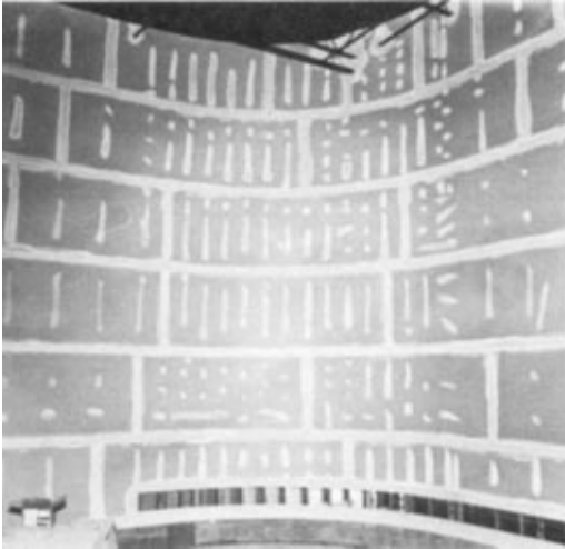
A tall backdrop of studs and board for a mockup of the Gulf of Mexico. Oil drilling rigs will follow.
