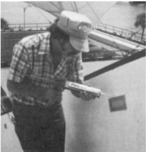
Here sealant is being applied on the perimeter from a tube vs. bulk application.
