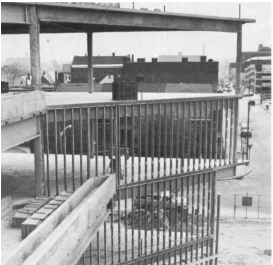
Exterior walls around the entrance to the Erie Insurance Group building were framed with pre-cut Cee Studs. A brick bearing angle is visible above the sheathing on the first floor frame.
