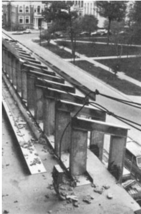
A close-up of the inverted “J” framing sections on the fourth floor of the Erie Insurance Group building. Light gage steel track was power-fastened to the slab, and then the short end of the “J” section was placed in it. Erie Acoustical fabricated “J” sections from 4” and 6” Cee Studs.
