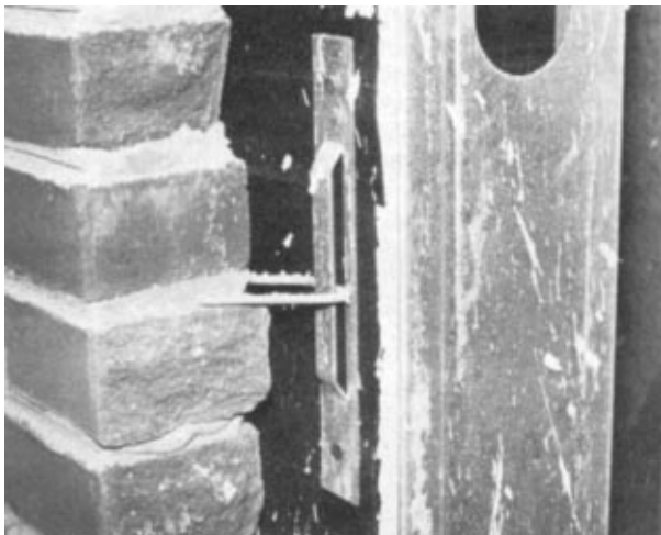
Masonry workers used screws to attach DW-10 adjustable brick ties to the 14 gage Cee Studs through the ½" gypsum sheathing.
