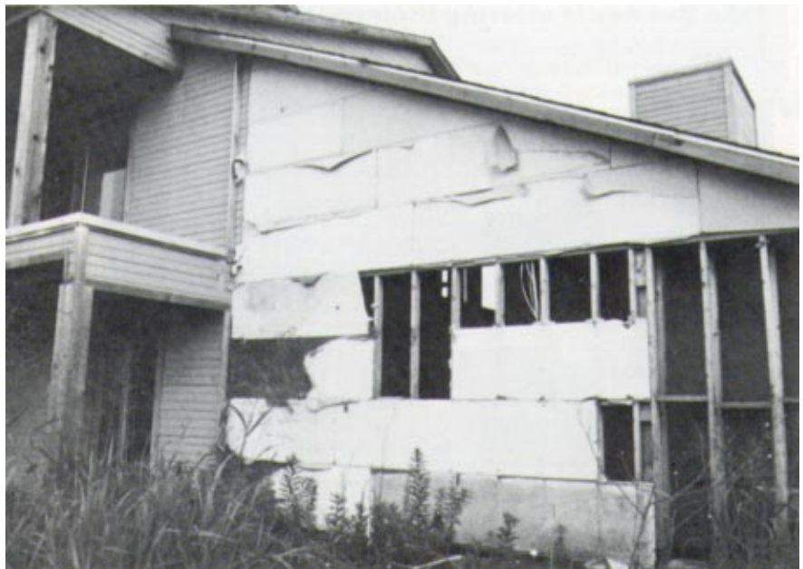
Failure due to long-term exposure to elements (over one year). Blow-off occurred due to over-driven and improperly spaced nails (12' o.c.). Sheathing protected under soffit area appears to be O.K.
