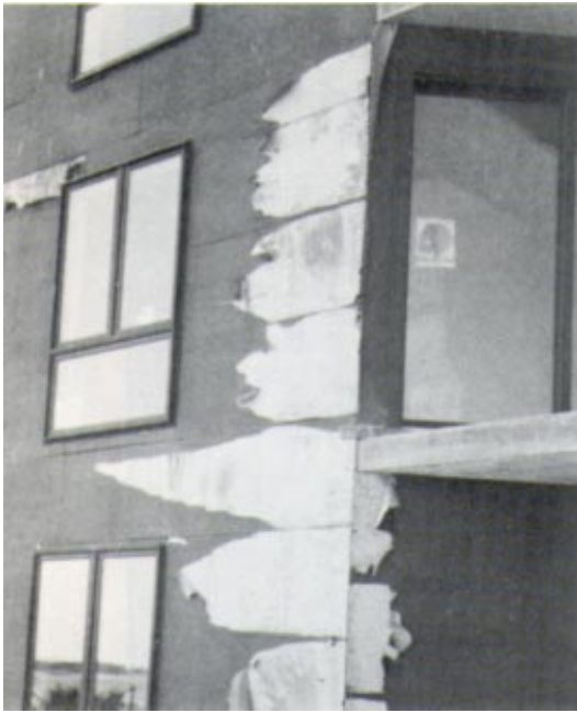
Severe winter exposure can create problems especially to unprotected ends and corners.
