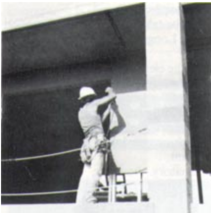
Drywall mechanic installing gypsum sheathing over steel studs for use as a base for a modified stucco system.
