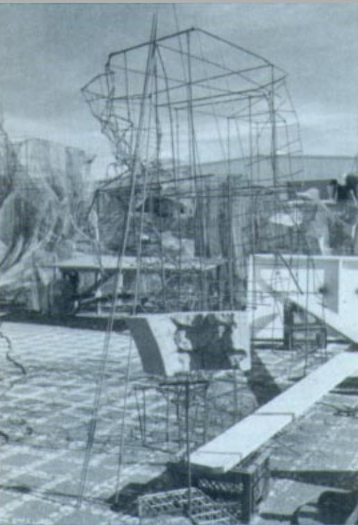
Forming is started on one of the 720 rock cages necessary to build Splash Mountain. The 1" scale model section in foreground is what craftsmen will follow to fashion the identical section in full size.
