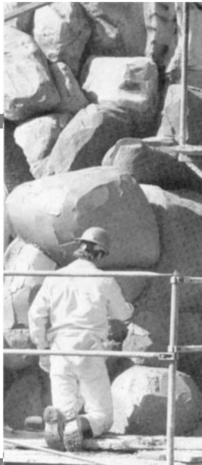
Plastering journeyman from The Bolster Company hard at work fashioning a tree trunk from plaster.
