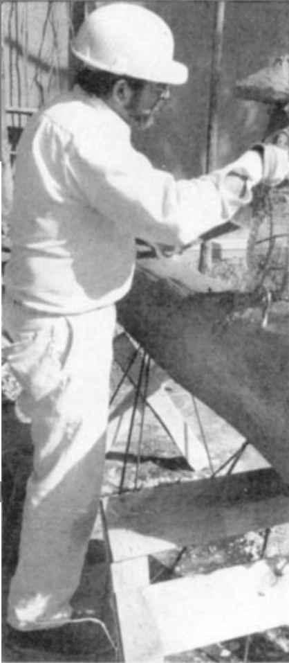
Plasterers hard at work sculpturing boulders at Splash Mountain. Painted circles on "rock" formation indicate where plaster protruding stones will be formed.
