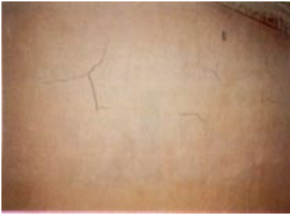
Deteriorated and cracked stucco surface.
