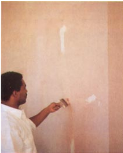
Hairline cracks in the surface are filled by brushing a smooth elastomeric into the crack and feathering the material.
