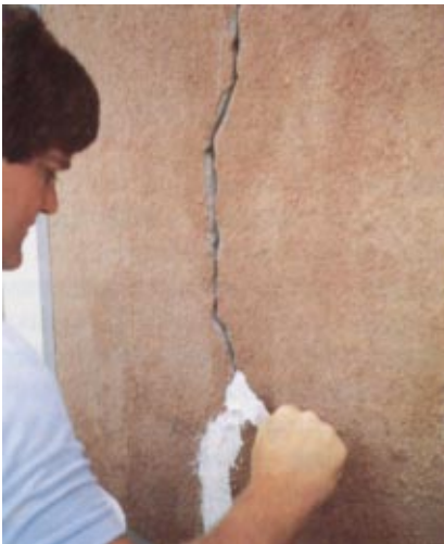
For cracks larger than 1/32", a knife grade elastomeric is used for the repair.
