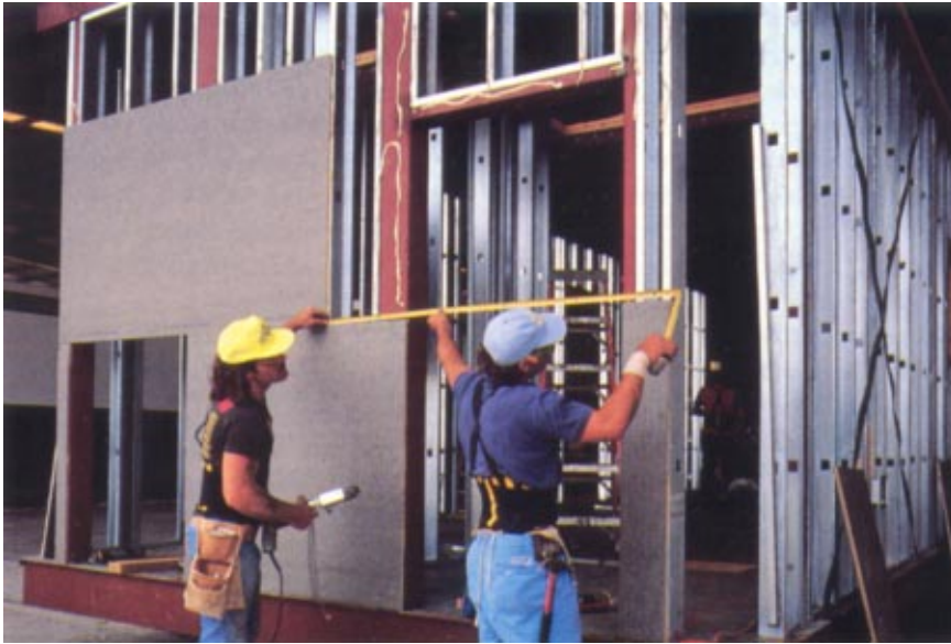
Highly durable fiberglass-reinforced prefinished (FRP) gypsum wall panels are installed in each unit.
