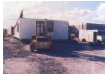
A crew of six men install a school building in just two days.
