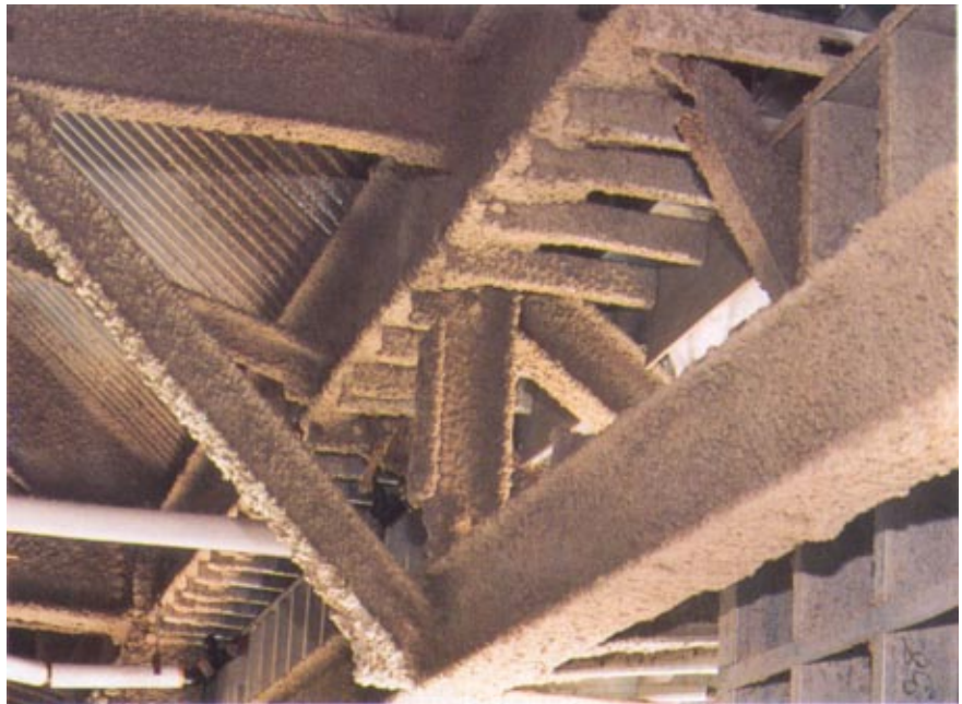
Much of the structural steel in the hotel's upper levels remained exposed to the weather during the extended timeframe required to install its complex sloped roof system. The use of a dry-mix product with UL listing for exterior exposures helped to minimize the potential for water damage.
