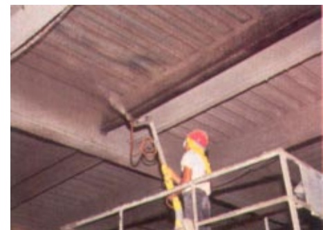
Above three photos: Scaffolding was used to apply the dry-mix fireproofing to the underside of the balcony seating area in the theater.
