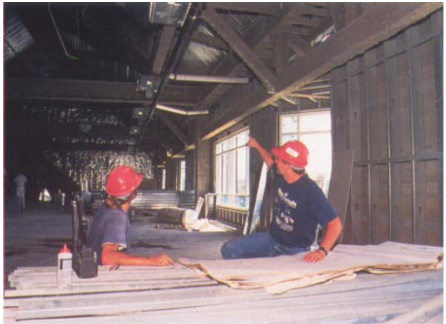
JESMAC Project Superintendent Tom Percell points out sections of the hotel's upper levels to be sprayed in the final stage of fireproofing application.
