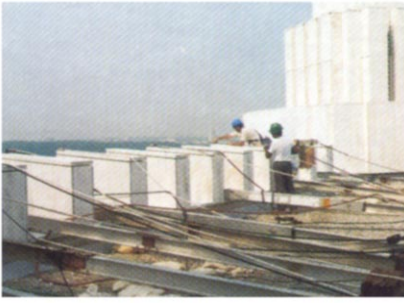
Workers check safety lines on the rooftop. Note the beams that counter balance the tow-man baskets, which are lowered between fin walls.
