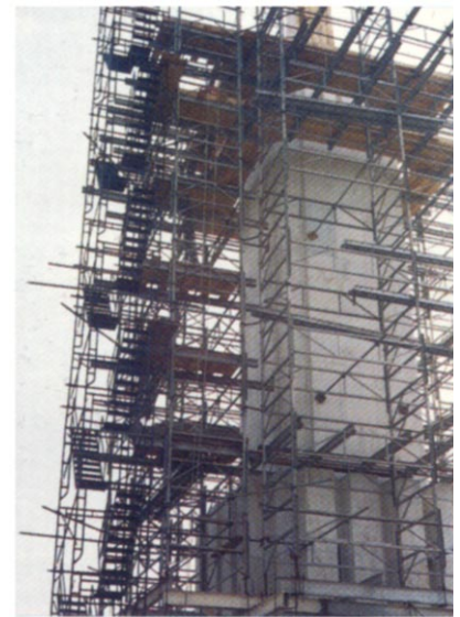
Scaffolding on one of the six towers rises from the roof to the base of the gold-plated spire. Photo by Kathy B. Sedgwick.
