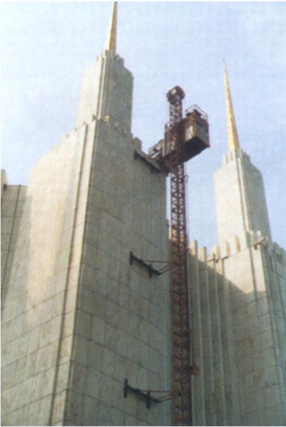
The hoist tower had to fit into a very narrow gap in the side of the building.
