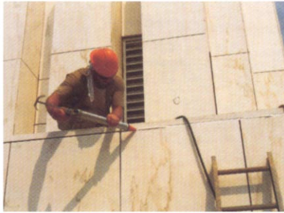
Bruce Carter (Pagliaro Brothers) adds new caulk to a horizontal joint on one of the six towers. Photo by Kathy B. Sedgwick
