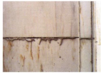
Deteriorated sealant has softened and melted out of horizontal joints. Photo by Kathy B. Sedgwick.
