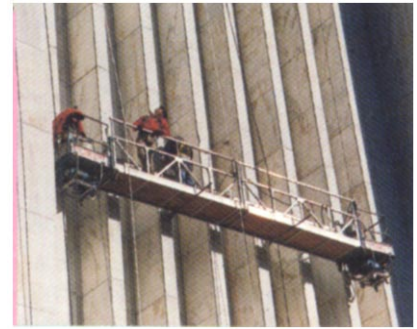
Narrow “fin” walls complicated the job. On the left a small “basket” rides beside a modular platform rigged to work outside the fins. Photo by Christopher Bates.
