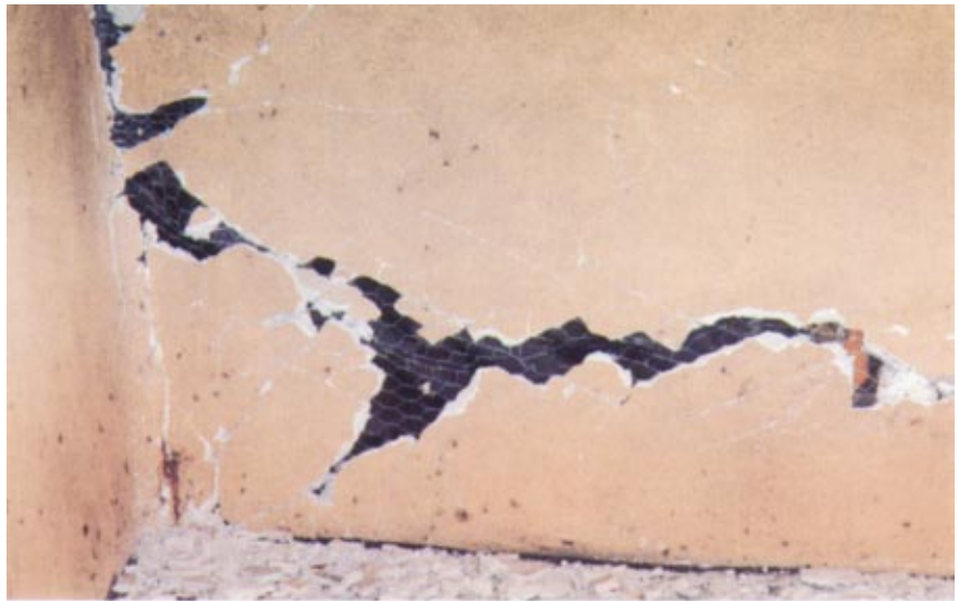
Extensive damage in Northridge earthquake showing stucco netting.
