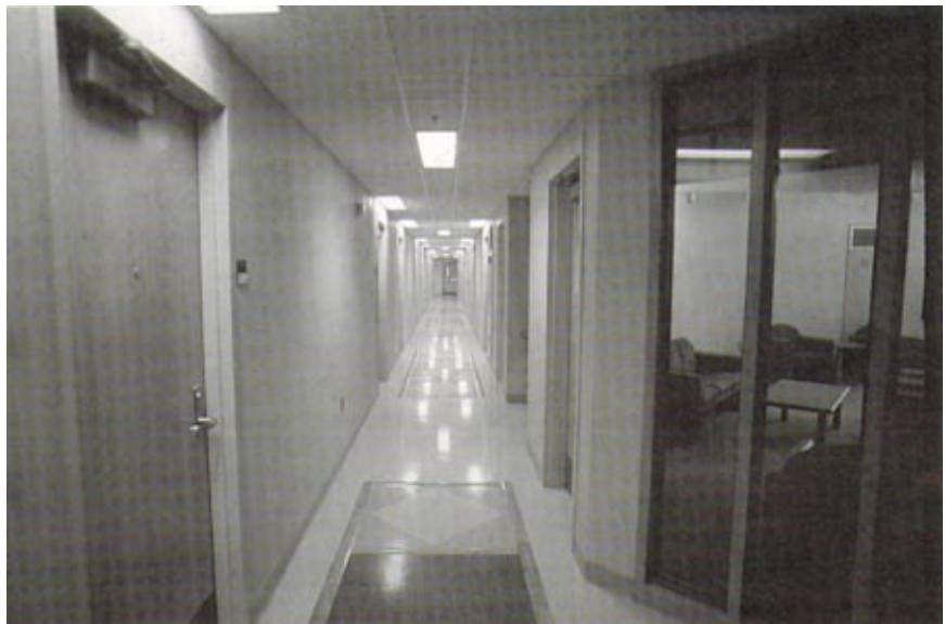
Veneer plaster system installed over cement board at Hillenbrand Hall on campus of Purdue University.
