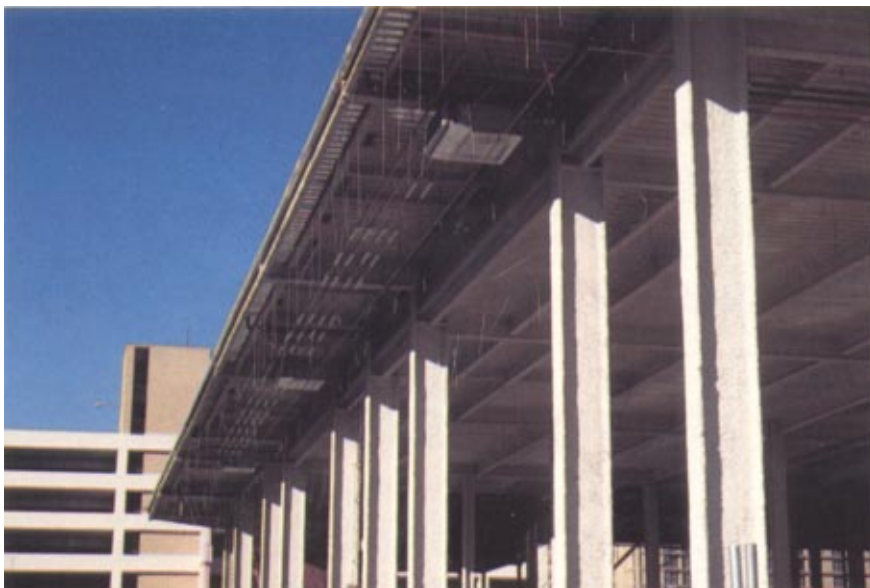
Retail space for several large tenants on the first three levels of the facility also required sprayed fire protection (Photo by Randy Stubbs, San Diego, Calif.)
