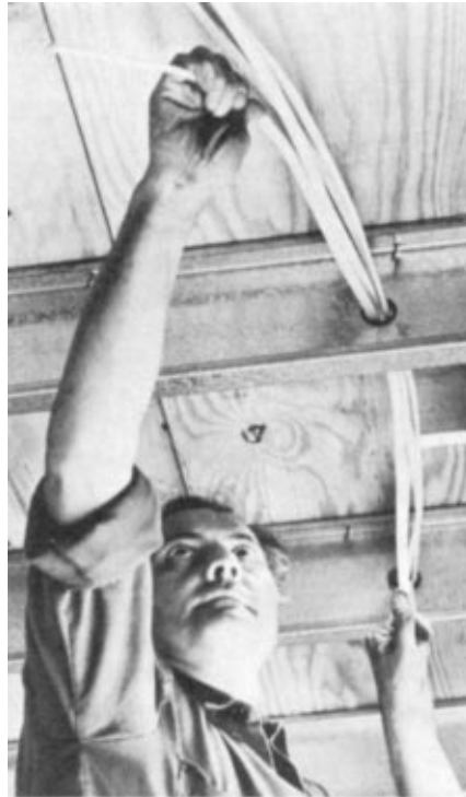
An electrician pulls wiring through pre-punched holes in steel joists. Some studs and joists have openings which reduce weight, improve heat transfer properties and help plumbers to install piping more easily.
