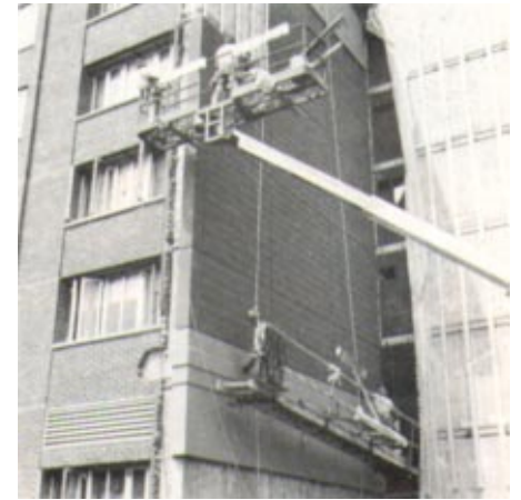
Workmen on aerial lift and swing-stage scaffold mechanically fasten lightweight Fedderlite Panel Systems to senior citizen center in Newport, RI. Brick cladding was removed, exposing concrete sidewall.
