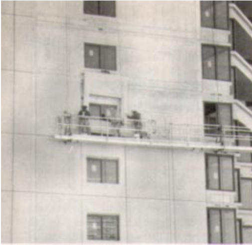
Workmen on swing-stage scaffold positioning Metalite Panel Systems on The Rittenhouse at Rittenhouse Square, Philadelphia, PA.
